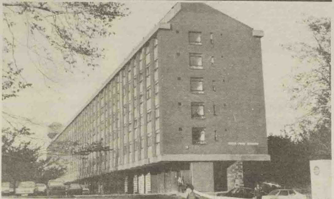
The Polytechnic Fine Art building has been closed after lumps of glass fell from the top of the building.
