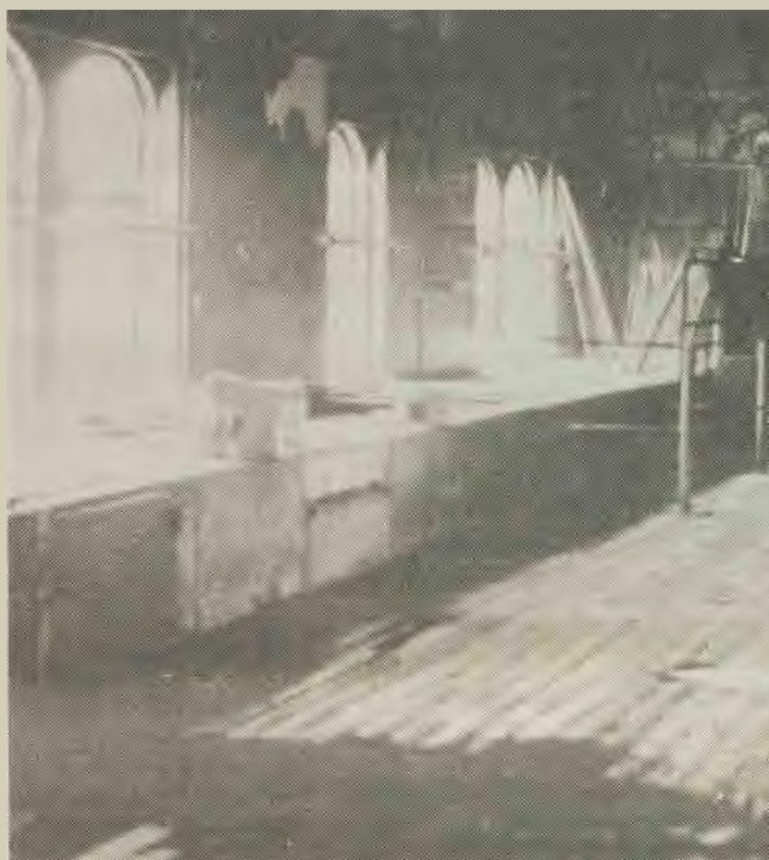
• Cosmo club's gutted interior
