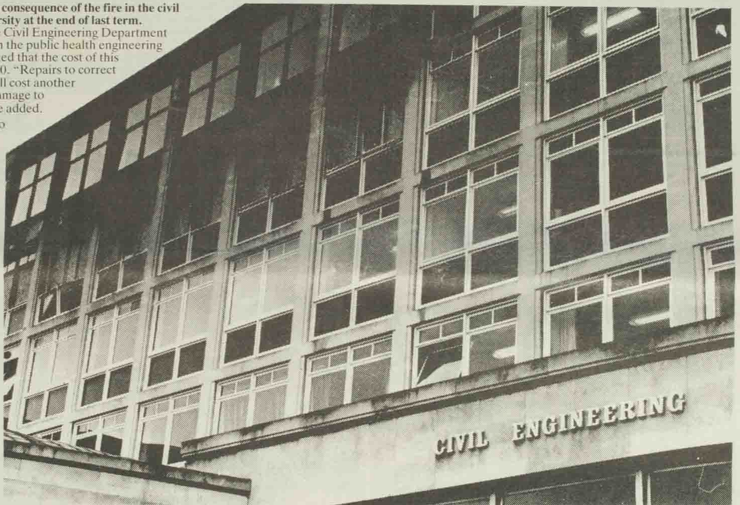
● The charred remains of the fire ravaged civil engineering building.
