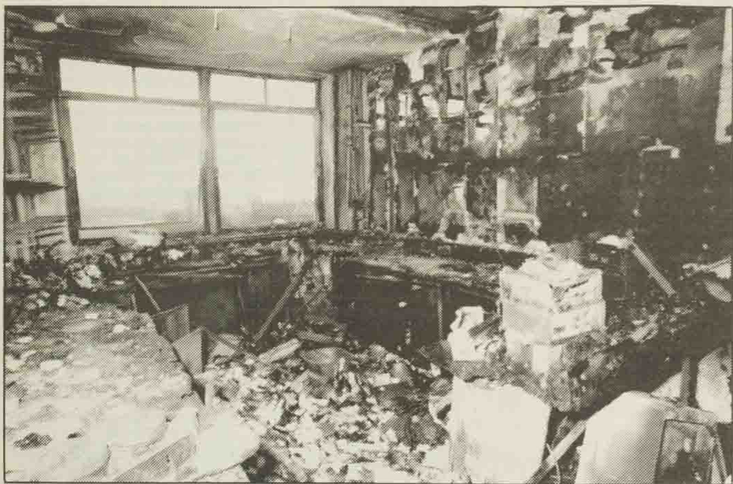
● The morning after the night before – a shattered civil engineering building, 12 hours after the explosion.
