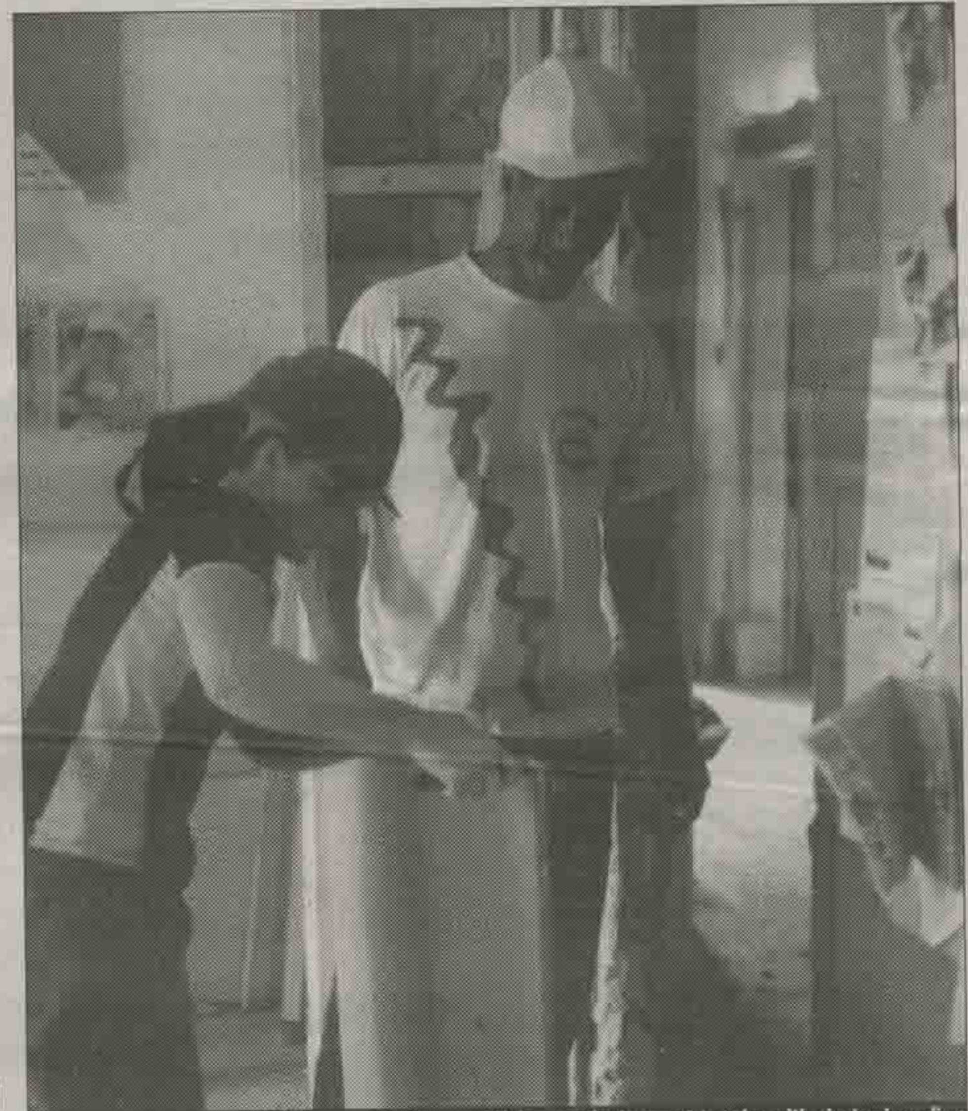
Brisco, a self-builder, and Helen, a volunteer, get to grips with plaster-boarding
