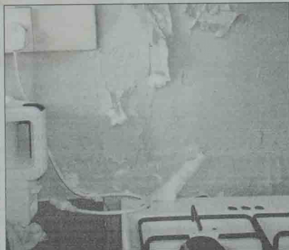
DODGY WALLPAPERING: The daily view for some tenants
