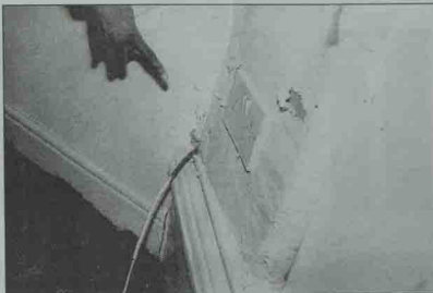
DANGER: A student points out the electrical problems in her house
