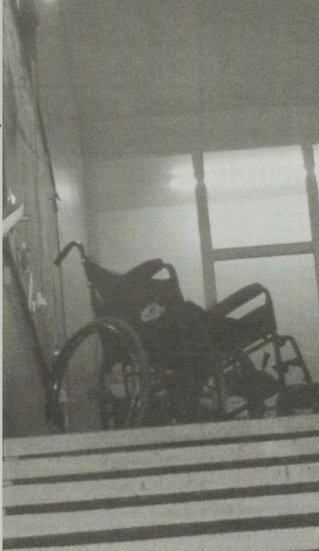
ACCESS DENIED: The lift for disabled access in both unions has been out of order PHOTO: JES SALTER
