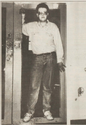
Emergency exit - broken fire door in Beckett Park.
