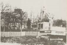
The cause of the noise at Clapham Park, Bostington.
