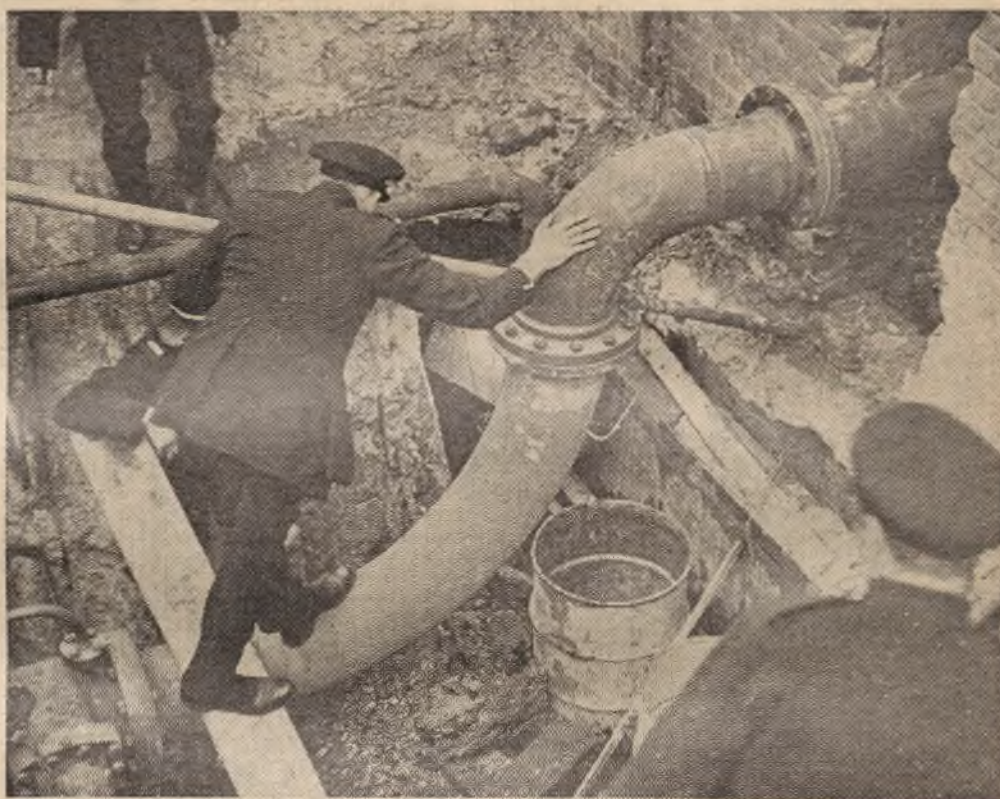
Firemen inspect damage after fire outside Arts Block
