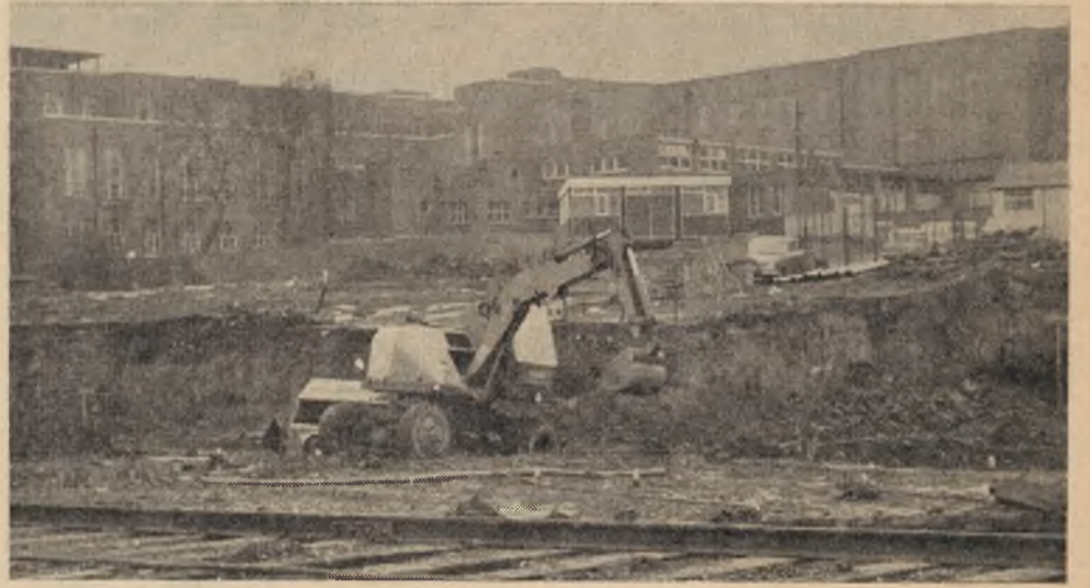
This view of the Union, from Virginia Terrace, will soon disappear. Work on the new maths/geology block is moving apace. When it is completed, it will hide the Union from sight—till the 2064 demolition squads start work!
