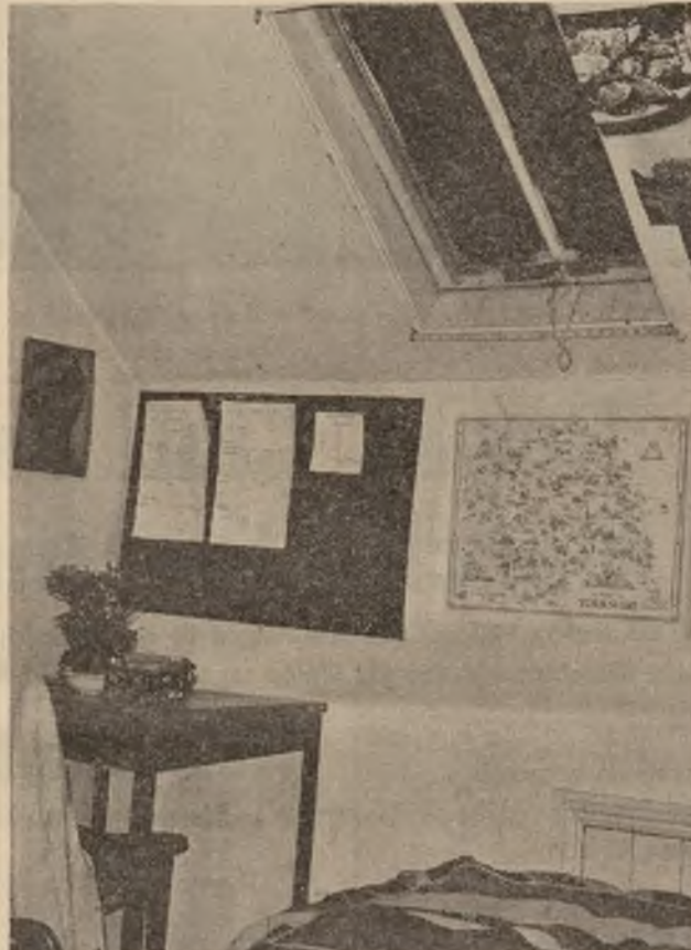
This window, taken from a student flat, is an example of not complying with health regulations
