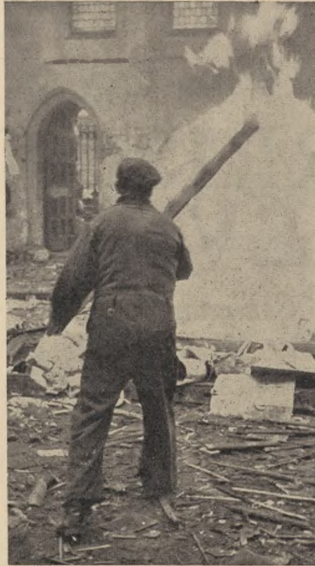
On all sides of the University demolition is in progress. Now, Lyddon Church, long used by Union societies for storage purposes and for ball decorations, comes down. The question now facing ball organisers is, where can they make their decorations?
