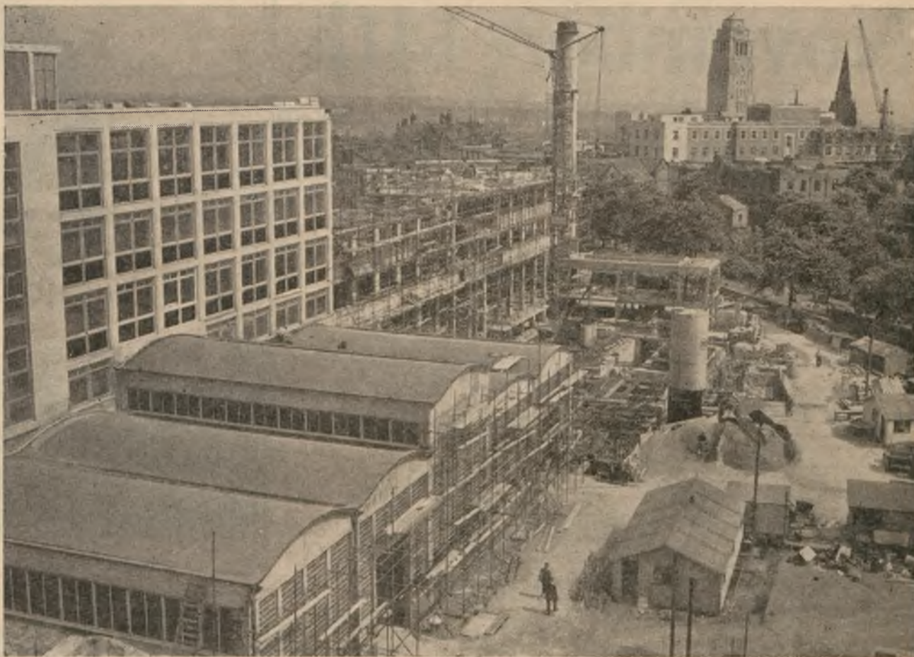
One of the major achievements of the Sixties was the building programme. The Engineering block is here under construction.
