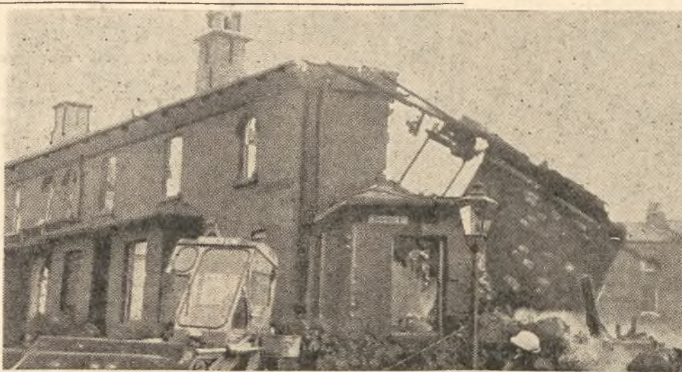
Another slum house crumbles to dust as demolition proceeds on Virginia Road. This is the site of the Charles Morris Hall of Residence due to be started in the New Year.
