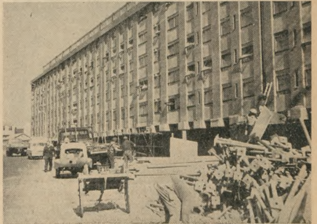
The Henry Price Building ten days before opening time. Though still not complete, there should be no major inconveniences to occupants.
