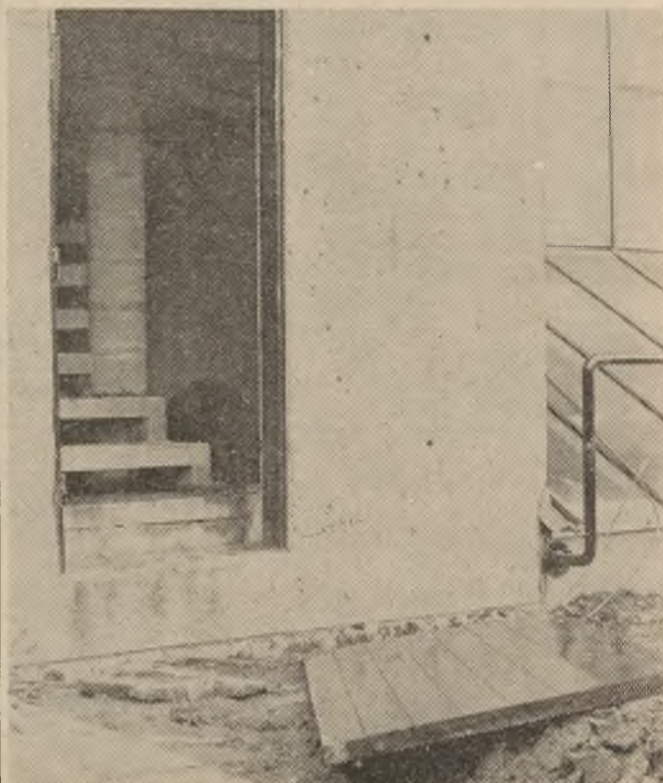
The smashed door in the Union Extension
