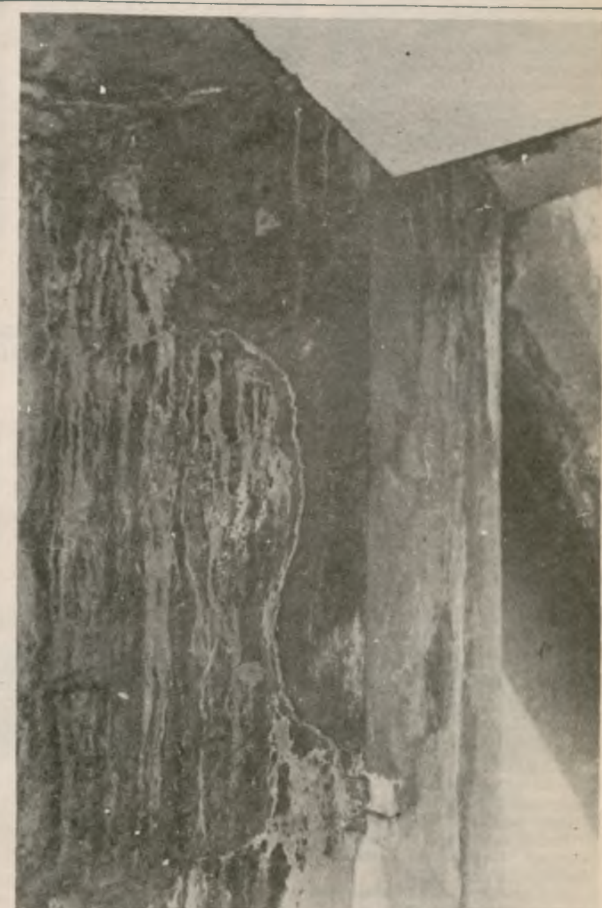
The picture above shows another crack below the steps leading up from Chancellor's Court past the Maths/Geology Block to Charles Morris Hall. Again, there is considerable staining due to water penetration.
