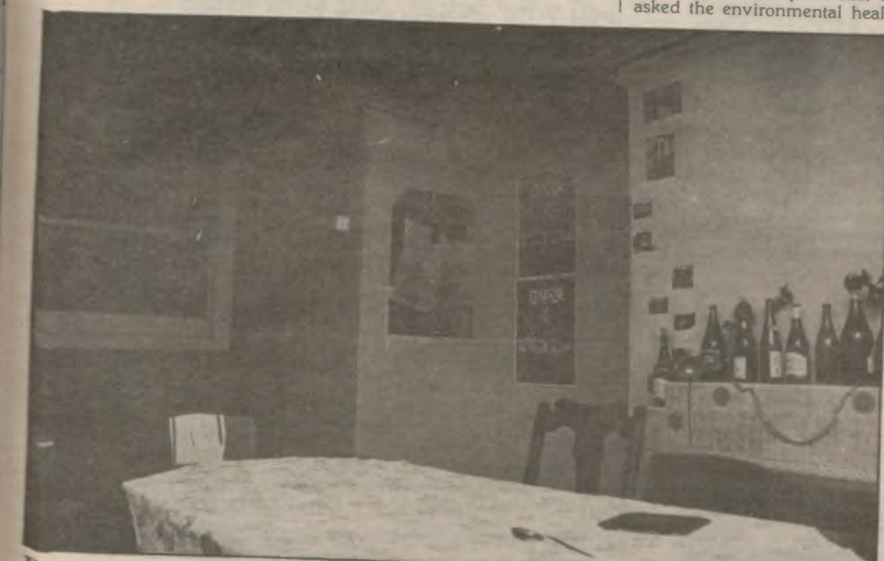
Basement of a house on Brudenell Road. The tenants pay £9 a week all year round. The rent office assessed a similar house at £153.90 per calendar month.
